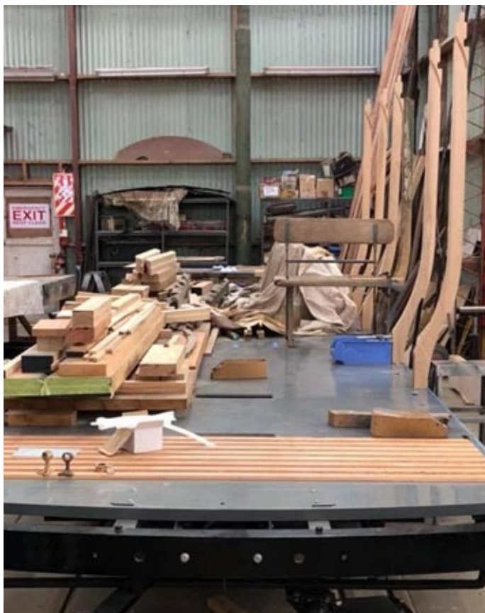
ABOVE: A trial fitting of the side pillars and their hold down brackets into slots in the frame, before to ensure everything fitted before final finishing.
